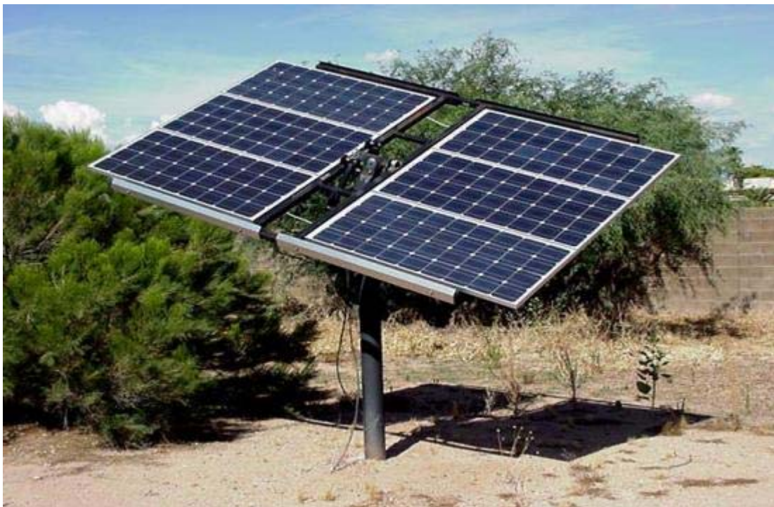
Figure 15 Photovoltaic modules with active monitoring of the Sun motion, Tracker
